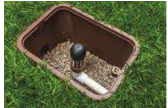
Air/Vacuum Relief Valve Installed
