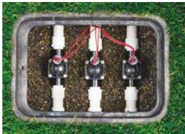
PGV-100G Valve Installed
