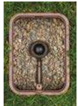
Automatic Flush Valve Installed
