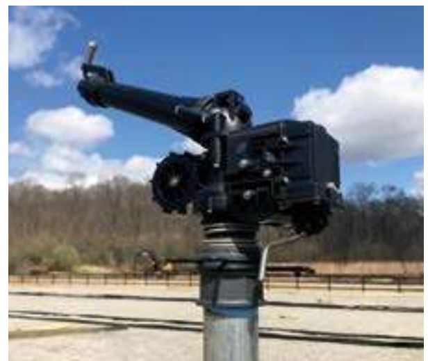
ST-1200-BR Rotor Installed
